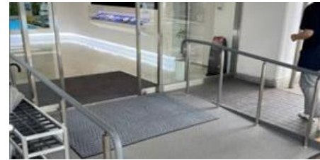
Increasing attendance rates by reducing the burden of movement through the installation of a ramp at the entrance.
