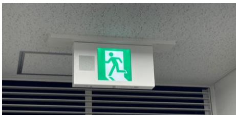
Improving peace of mind during emergencies with the installation of flashing emergency guide lights with audio guidance, enabling situational awareness through both sound and light.
